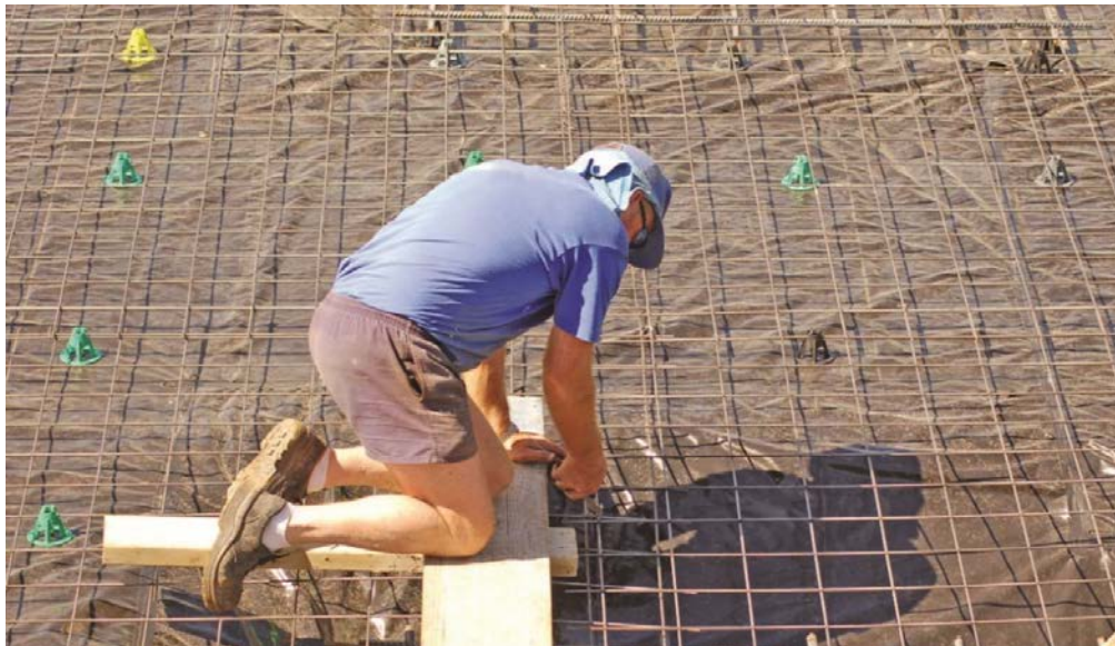
Standard construction mesh being placed into position before concrete is poured (plastic supports are used to keep the mesh elevated).
